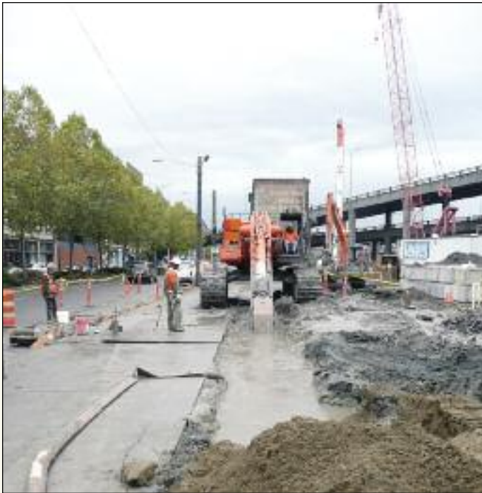
Figure 3a and 3b below – Pre-trenching under cement-bentonite slurry to remove obstructions to 30 feet depth.
