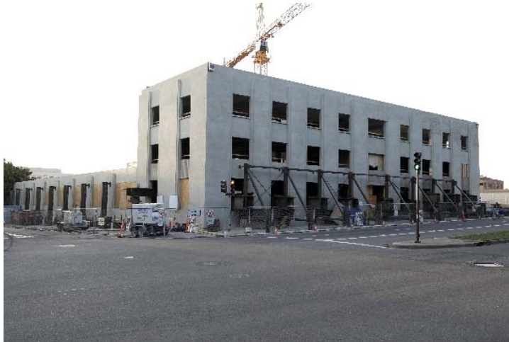
Figure 9. Buttresses Bracing the Admin Block from Outside the Site (Photo by Degenkolb Engineers)
