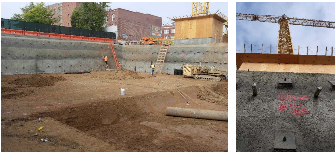
Figure 5 (left). Soil Nail Bulkheads at Completion of Excavation Figure 6 (right). Pre-Loaded Soil Nails w/ Angled Anchor Head (Photos by Degenkolb Engineers)
