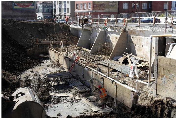
Figure 7. Existing Parking Garage Wall Braced by Concrete Buttresses (Photo by Degenkolb Engineers)
